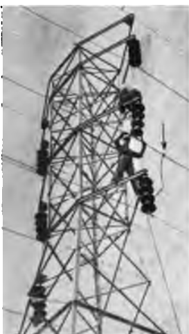
Fig. 7. Ground Connection on High-Tension Tower.
